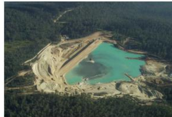
Fig. 2. Work in progress to implement a water cover for the Benambra (Victoria) tailings dam
