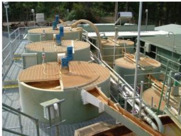
Fig. 4. High density sludge lime neutralisation plant at Brukunga (South Australia)
