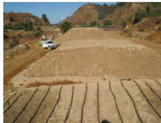
Fig. 1. Setup of field test pads to evaluate high alkalinity producing cover designs at Brukunga, South Australia
